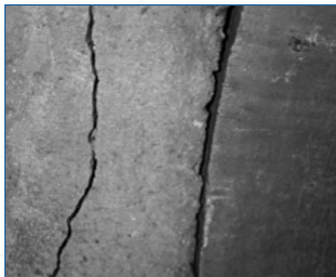
Figure 8: Crack Width Exceeding Design Crack
