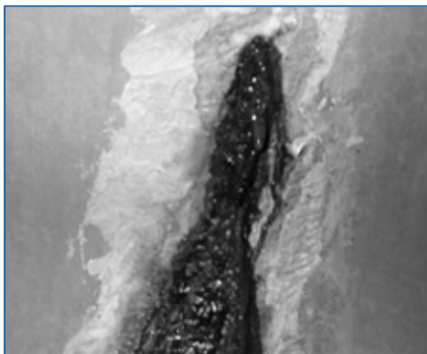
Figure 9: Dynamic Crack Not Showing Positive Autogenous Healing Effects
