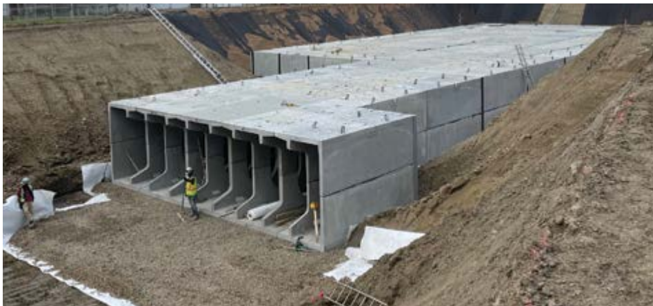
View of entire installation layout
