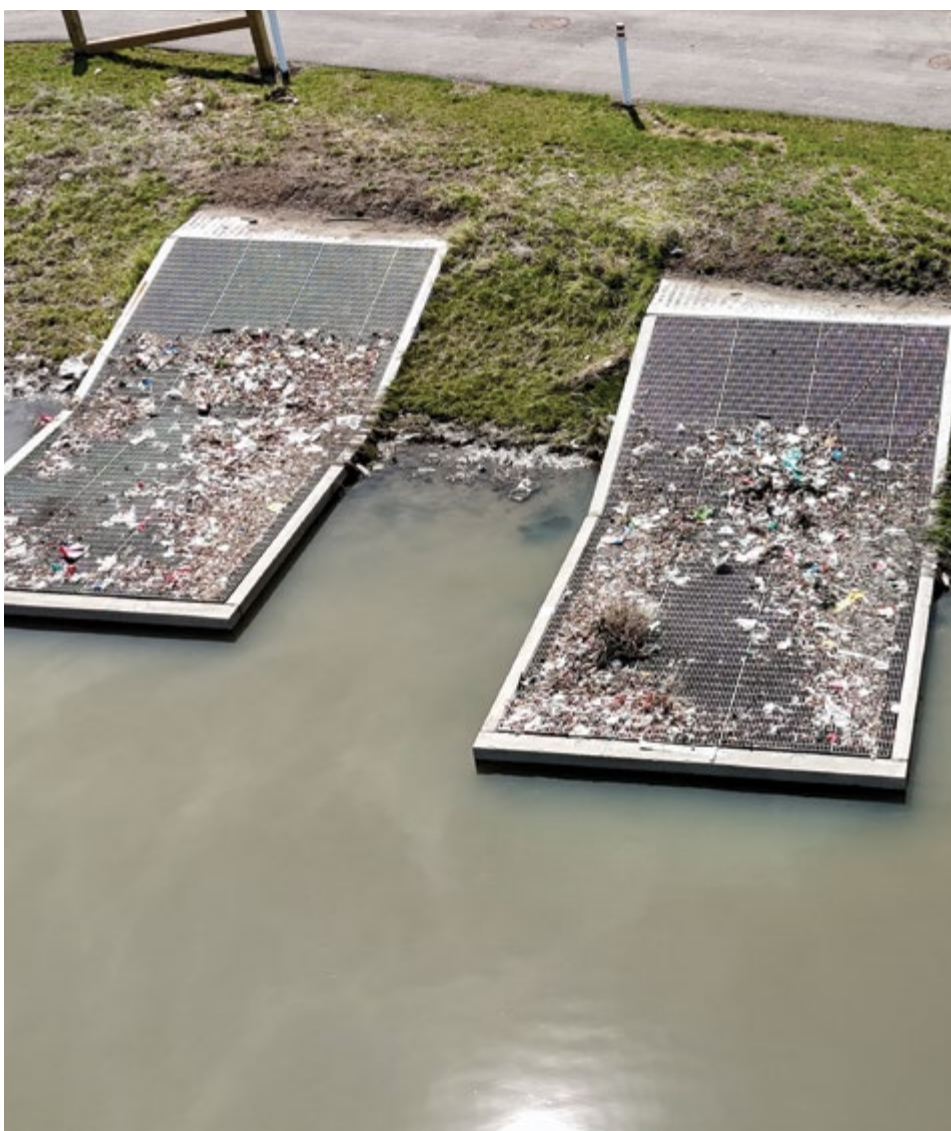
The finished Nautilus Pond® outlet structures capturing floating debris and protecting the Bow River
