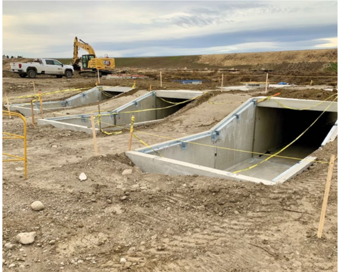
Precast Concrete Box structures are installed at the outlet of the Nautilus Pond®
