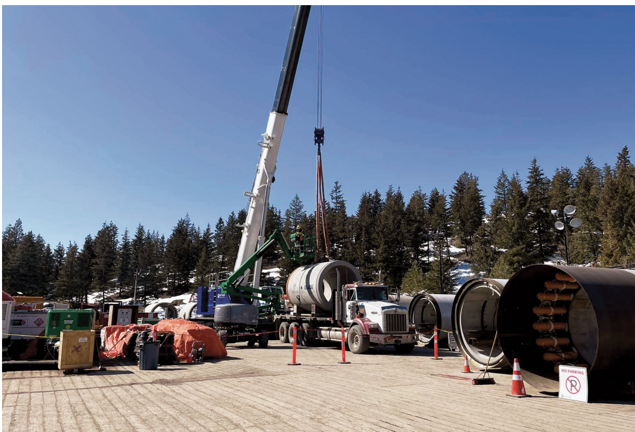
Reinforced Concrete Jacking Pipe (RCJP) being loaded on a transport vehicle and an Intermediate Jacking Section (IJS) is visible in the foreground on the lower RHS.
