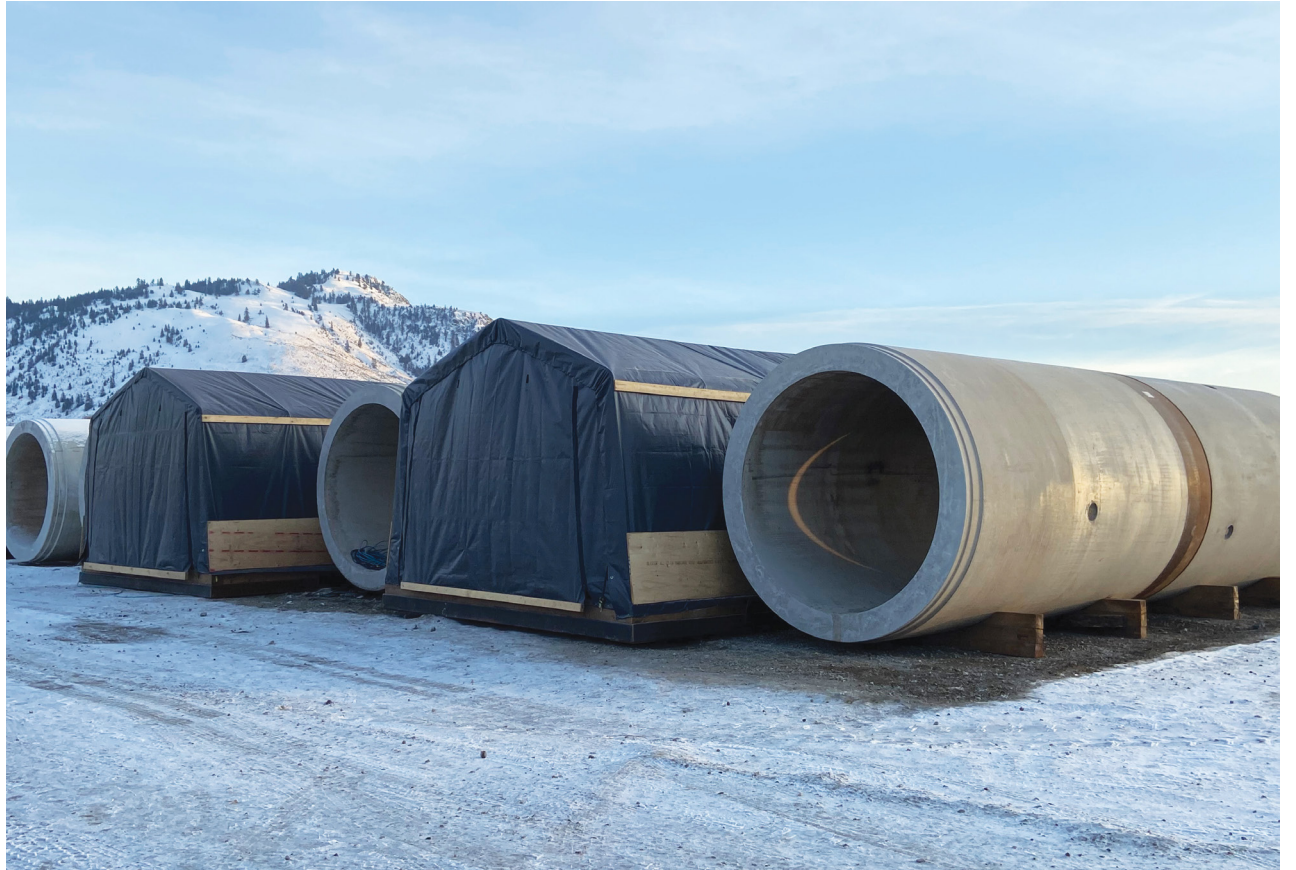
Reinforced Concrete Jacking Pipe (RCJP) in yard storage and some tented for steam curing.
