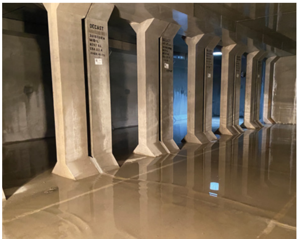
Picture 3: View of the installed I-STORM interior
