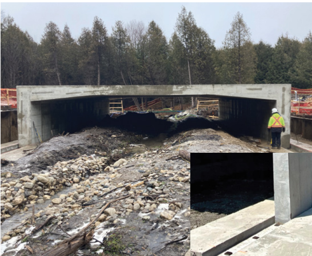
Installation of three-sided structure. Shim packs can be seen in footing keyway on RHS
