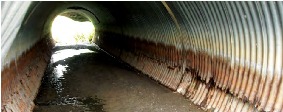
Complete section loss of existing CSP
