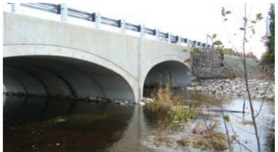
Completed structure with gabion basket wing walls, 0.3 m rip rap to armour the footings, and 100mm and larger cobble for the southerly dry channel and stream bank.
