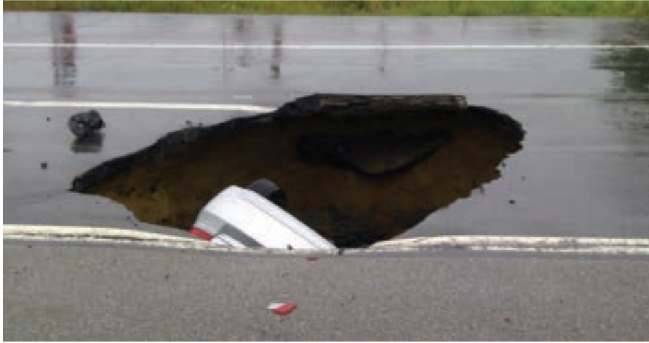
Highway 174 Collapse, Ottawa – Sept. 2012 Courtesy: Ottawa Fire Services
