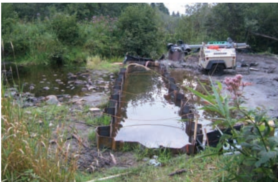
Footings prepared for CON/SPAN system designed to CAN/CSA-S6-06, CL-ONT-625 to accommodate stream flow, runoff and local traffic.
