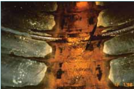
Cracked HDPE Liner.
