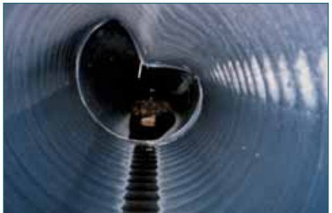
Failed Pipe Wall Buckling.
