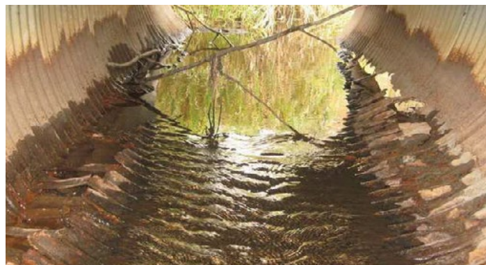
Rusted CSP culvert in service under busy Ontario highway
